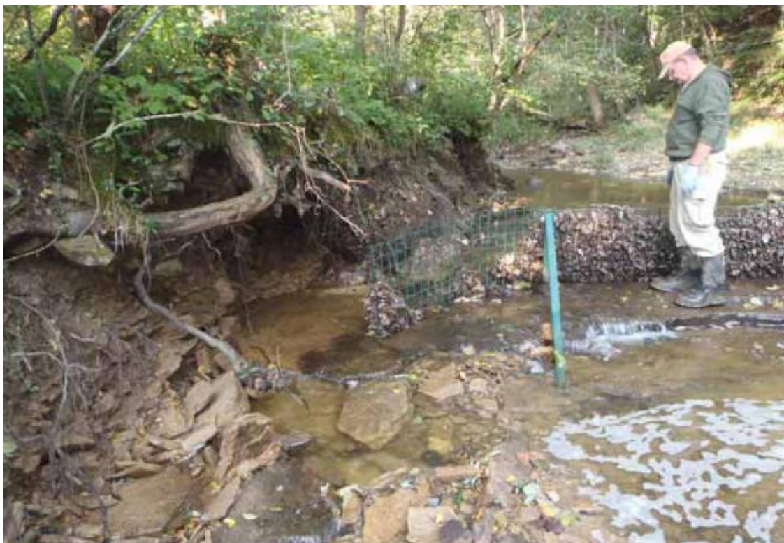
PICTURES SHOWING EROSION OF STREAM BANK NEAR SOUTH END OF BARRIER
