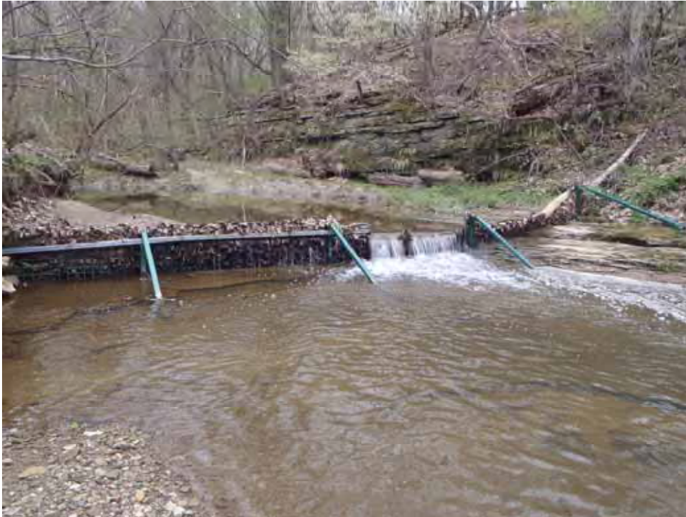
PICTURE SHOWING BUILD UP OF DEBRIS ON BARRIER.
