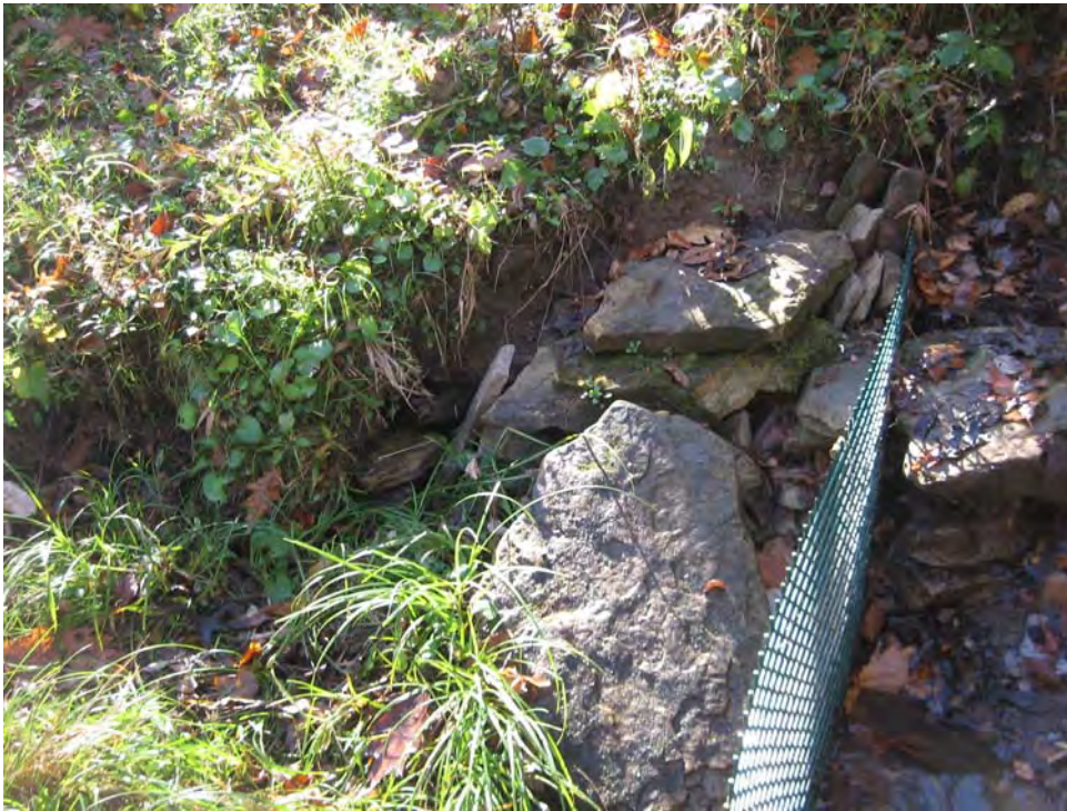
Washout area at barrier
