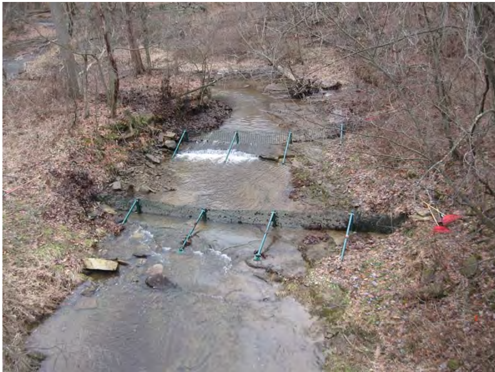
Overview of barriers following cleaning operations. Note: Remaining debris seen on screens is frozen to the screens.
