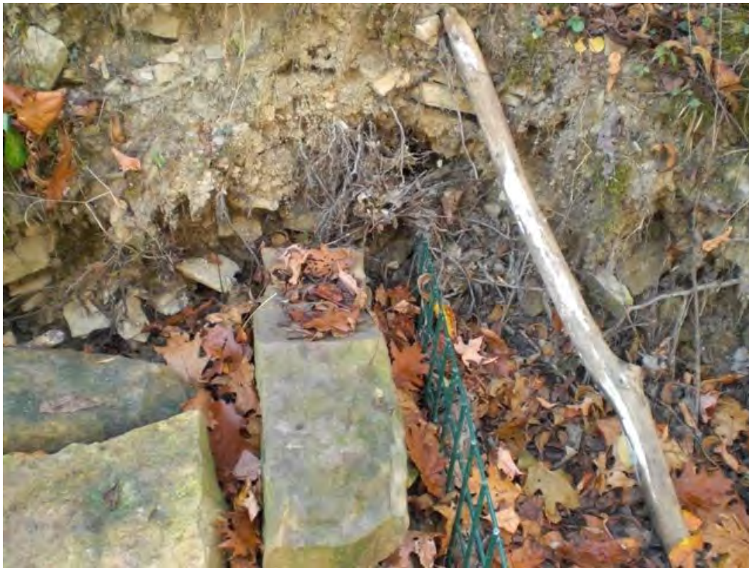
Photo 5: Scouring at south end of upstream (3-inch grid opening) barrier
