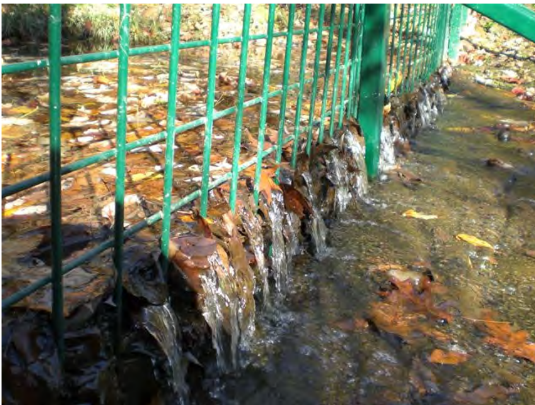
Photo 4: 7 – 8-inch deep leaves accumulated on the screen
