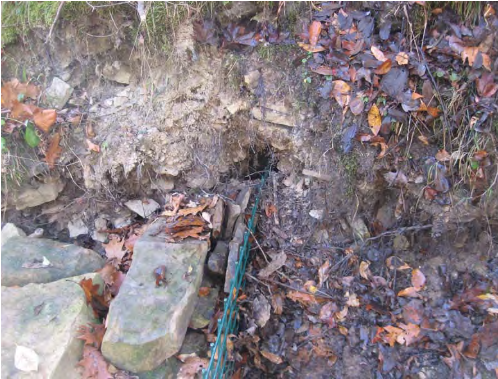
Washout area at barrier
