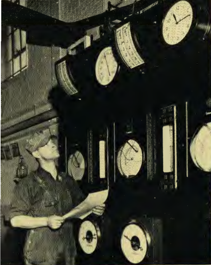
Frank Ticknor, fireman, takes readings from the gauge board of an oil burning unit. The instruments register steam pressure, the water level in boilers, oil pressure, and the daily flow of steam.
