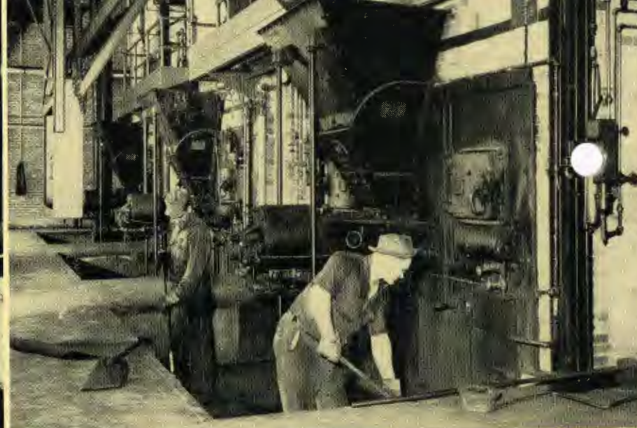
These are three of the coal burning boilers in Power Unit 3. Kenneth Stevens, fireman (left), and Harry Sheets, engineer, clean waste coal from pit in front of boiler.
