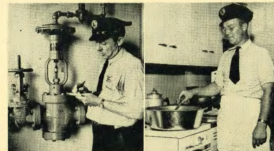
Upper left: Fire Inspector Victor Hoover, checking control on sprinkler (deluge) system used in operating buildings throughout the plant.
