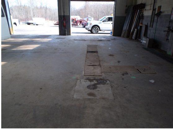
Photograph 2: Hydraulic lift and oil water separator vault in the floor of Building 1034. Photo facing East from Southeast corner of inside Building 1034.
