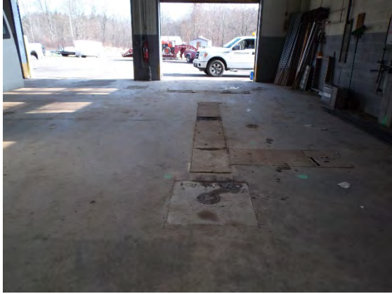
Photograph 2: Hydraulic lift and oil water separator vault in the floor of Building 1034. Photo facing East from Southeast corner of inside Building 1034.
