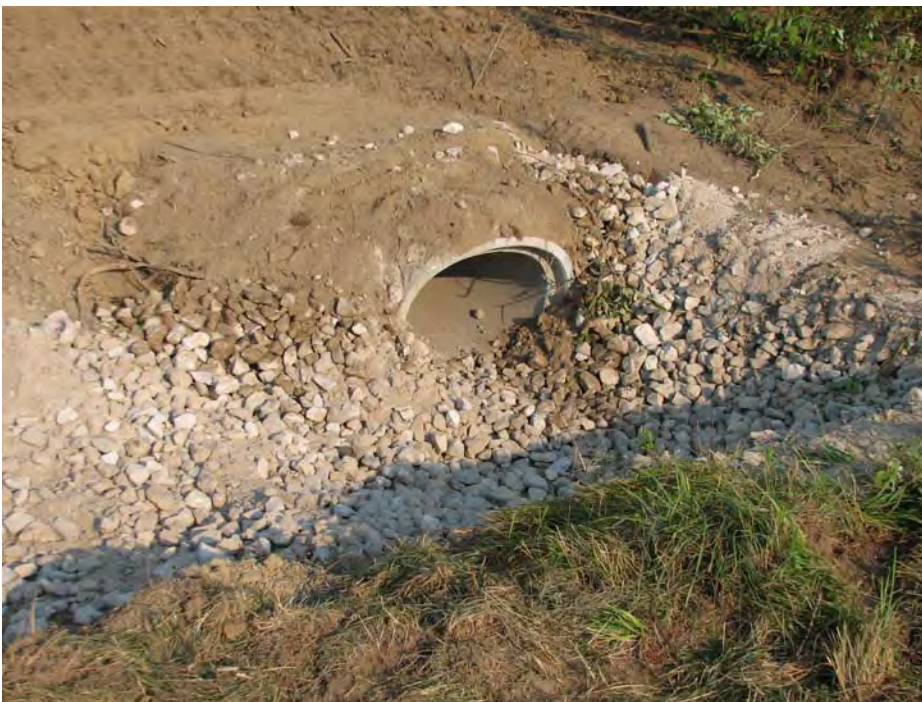
DLA East Ore Yard Site. Installed 24x36-inch elliptical concrete pipe and stone apron.
