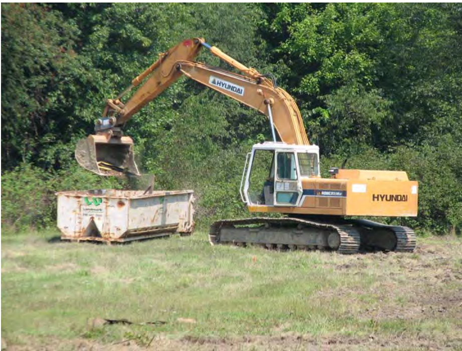
DLA Rt. 80 Tank Farm Site. Cleaning site of debris from previous operations.
