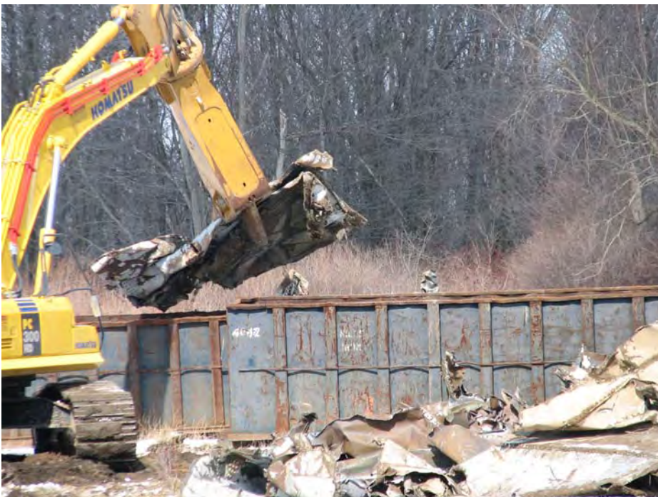
DLA Rt. 80 Tank Farm Site. Loading AST steel into dumpster for recycling.
