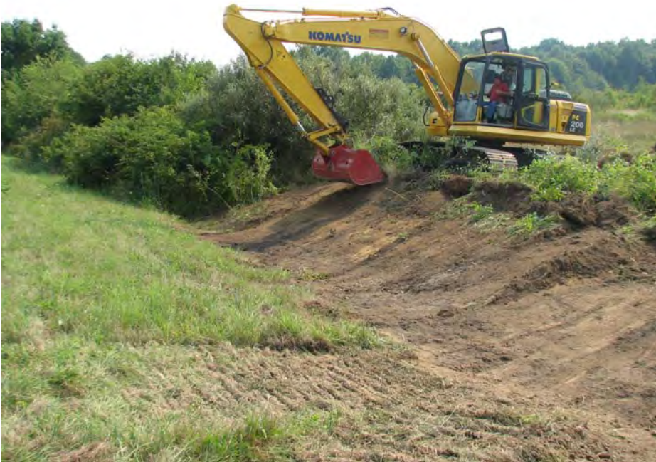
DLA East Ore Yard Site. Excavator clearing drainage ditch along South Service Road of vegetation.
