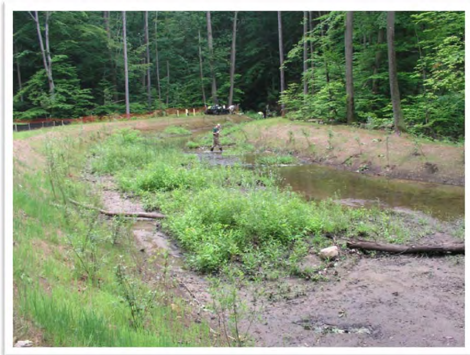
Photograph 4 (July 2, 2013) This is a view of the relocated stream channel facing downstream. Shrubs and aquatic macrophytes are beginning to establish.
