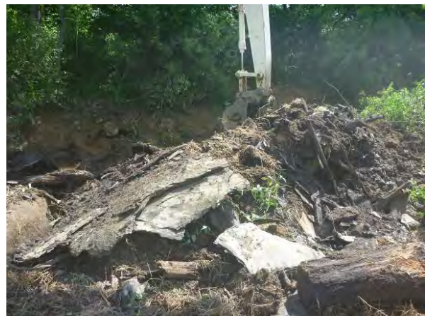
Photograph 3-6. Soil Containing Construction Debris
