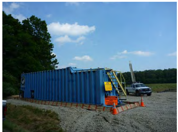
Photograph 3-2. Portable Water Storage Tank
