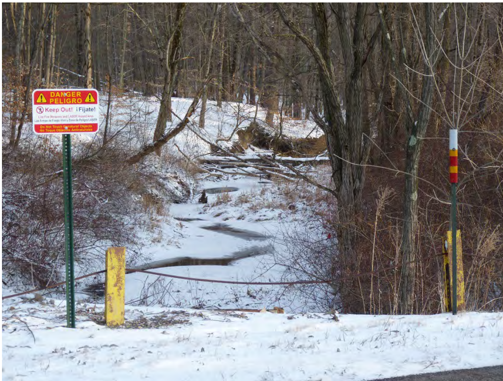
Open Demolition Area #2. Seibert stakes and warning signs along Newton Falls Road.
