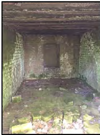
INSIDE CHANNEL FROM MAIN DOOR Note: The material beneath the grate in the channel has not been sampled.
