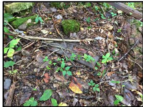
STEEL PLATE DOOR - BURIED
