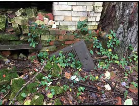
DONELLY CLEANOUT DOOR Note: The metal debris, including the cleanout door and steel plate door, are on the ground surface in front of the channel opening.
